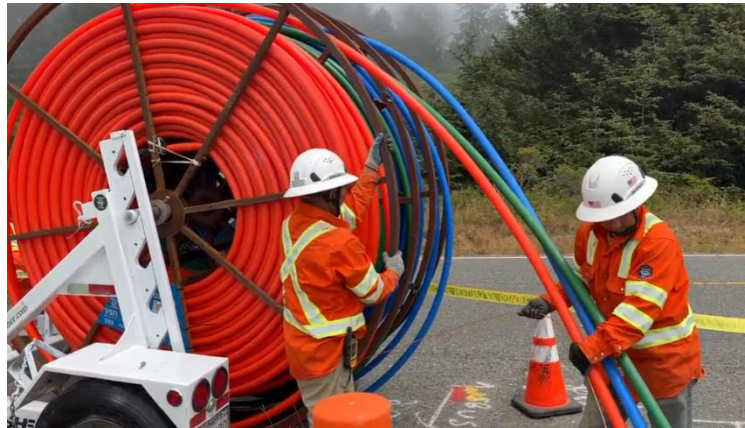
Figure 3: Vero Networks Construction workers assisting with pulling the fiber rolls through the ground.
