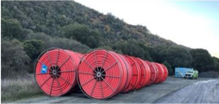
Figure 5: Spools of conduit at a state materials depot
